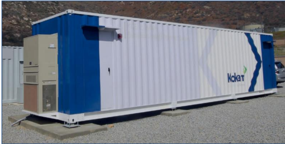
Figure 6: Kokam 40' Container BESS
